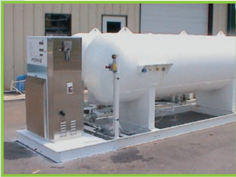
Propane is stored in above-ground tanks.
