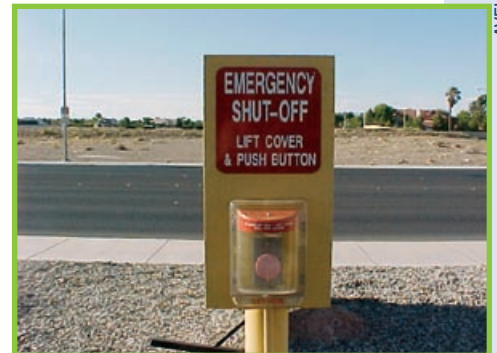
The emergency shutdown device stops the flow of natural gas to the pump. Drivers should take notice of the location of the emergency shutdown device at the stations they frequent.
