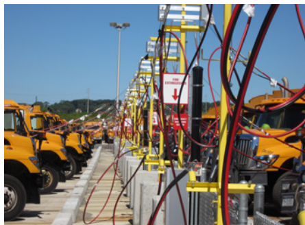
One of 21 CNG fueling stations in Oyster Bay available to local fleets of CNG vehicles. The CNG station was funded with help from the Recovery Act. Photo from Greater Long Island Clean Cities, NREL 23853
