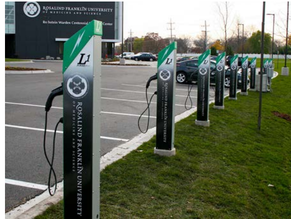
Photo 12. Level 1 pedestal EVSE at Rosalind Franklin University in Illinois. Photo from Telefonix.
