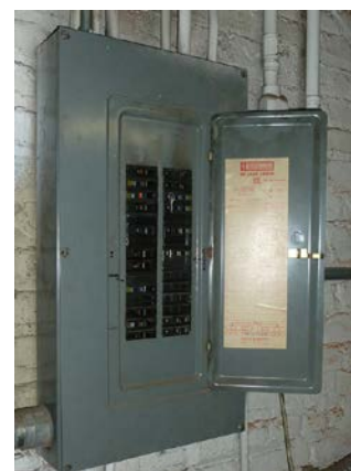
Photo 21. Electrical panel. Photo from NYSERDA.
