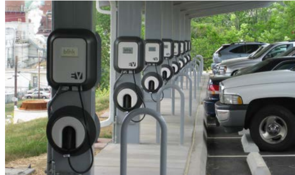
Photo 1. This series of Level 2 EVSE were installed by the EV Project. Photo from INL.
