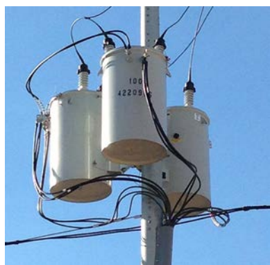
Photo 22. Step-down transformer located at the utility service point. Photo from Don Karner.
