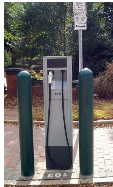
Photo 2. Pedestal-mounted EVSE installed by the City of Raleigh, N.C., for free public use. Photo from Kathy Boyer, NREL 18520
