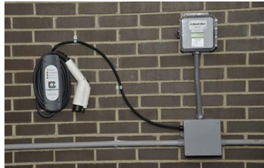
Photo 4. Wall mounted EVSE installed by the New York Power Authority for employee charging. Photo from NY Power Authority, NREL 26468.
