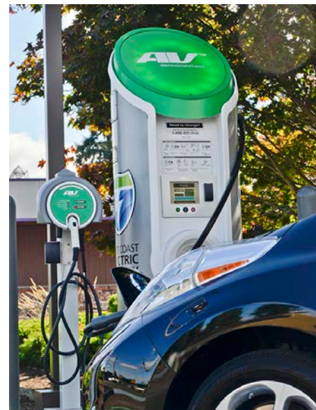
Photo 13. One of many side by side DCFC and Level 2 EVSE installed along the West Coast Electric Highway in Oregon and Washington. Photo from Washington State Department of Transportation (WSDOT).
