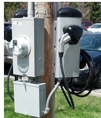
Photo 20. An electrical meter mounted alongside the EVSE and connected with conduit. Photo from NYSERDA.
