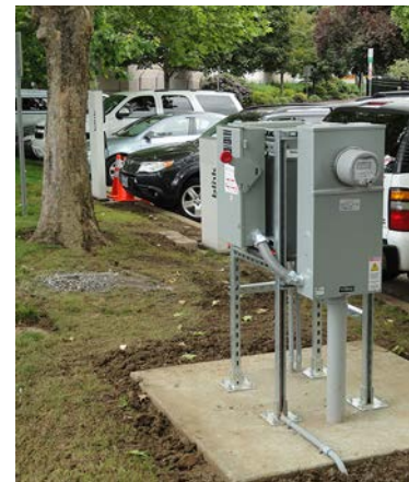
Photo 9. Electrical meter and switch servicing Level 2 EVSE. Photo from Don Karner.
