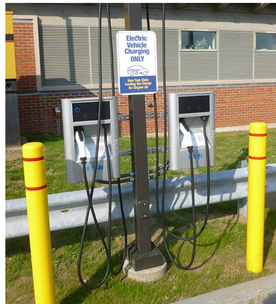
Photo 17. These two EVSE are located close to the building, reducing trenching costs. Photo from NYSERDA.
