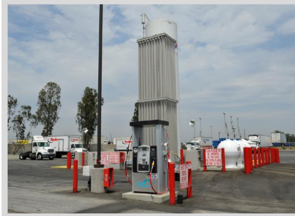
Figure 2. Ryder LCNG Station at the Fontana Maintenance Facility
