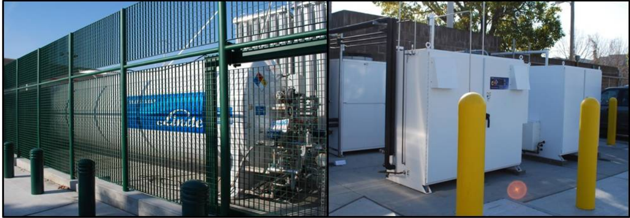
Figure 7. Emeryville station liquid hydrogen tank (left) and electrolyzers (right)
