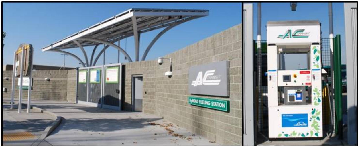
Figure 5. The light duty FCEV fueling access (left) and dispenser (right) at the Emeryville station
