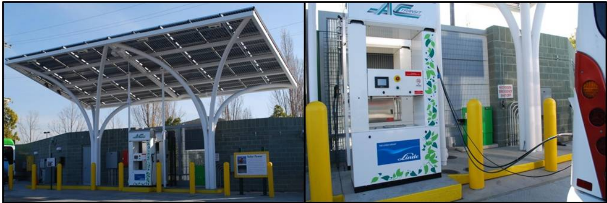
Figure 9. Bus fueling at the Emeryville hydrogen station: fueling area (left) and close up of the bus dispenser (right)
