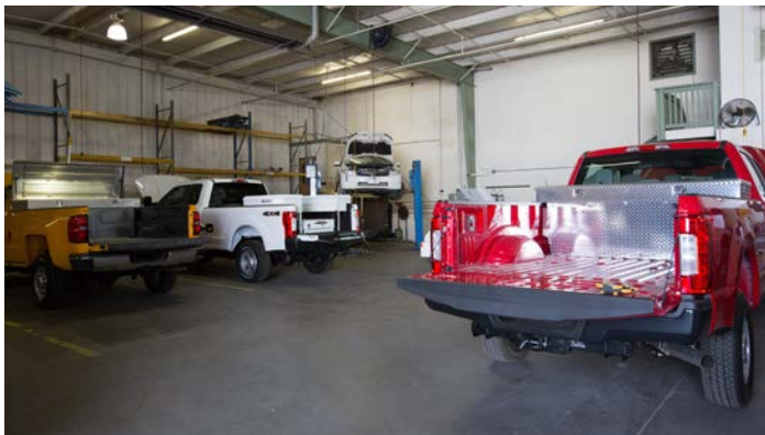
This CNG vehicle conversion facility is outfitted with a fuel-leak mitigation system. The system includes the in-wall exhaust fan shown in the upper right. Photo by Amy Glickson, NREL 45006
