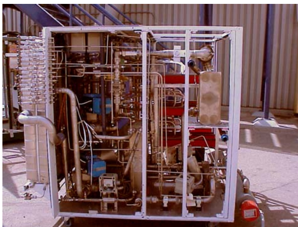
Figure 3. 50-kW brassboard system (without the stacks).
