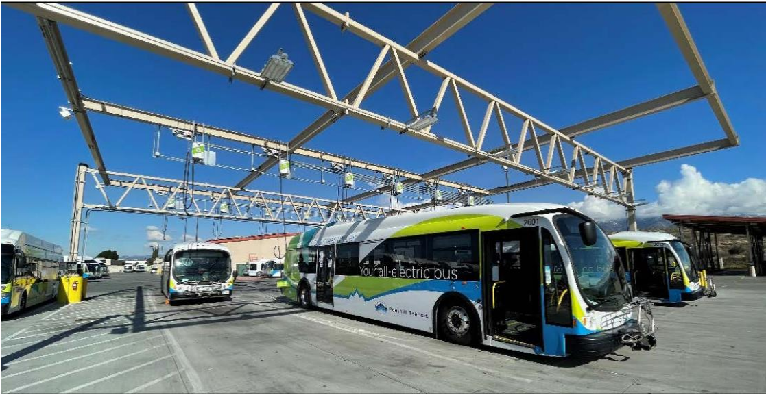
Figure 5: Plug-In Dispenser Cord Reels at Foothill Transit's Arcadia Depot
